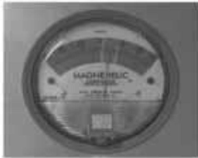
Image of room pressure gauge indicating colour coded normal, alert & action parameters
